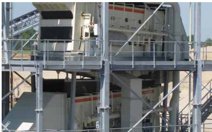
FS screens installed in cascade.
